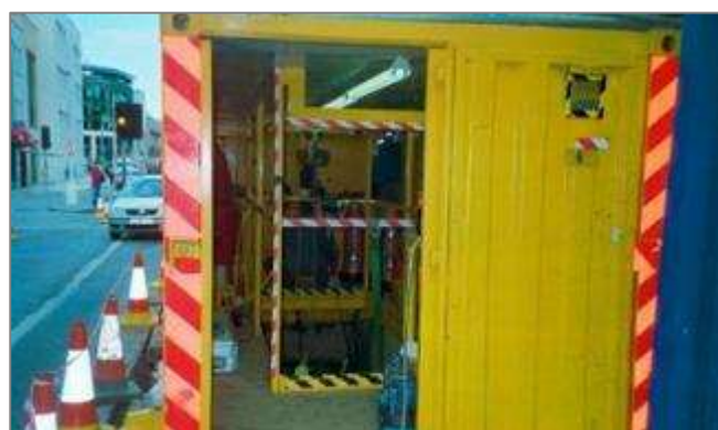
Figure 6: Cable Jointing Container
